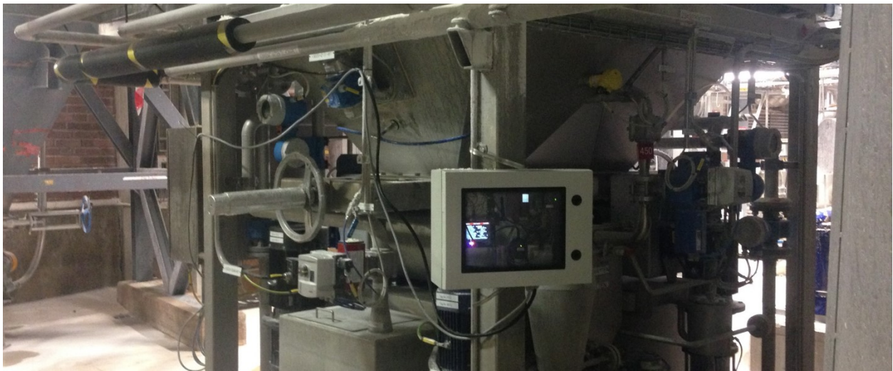
Figure 17. The environment where the wireless devices were installed. The picture shows a mixing tank where the flow of the slurry into the cooking process is measured. The gateway and the field devices were realized by assembling two off-the-shelf evaluation boards in an IP67 enclosure. A CAN bus IO from ABB (CI581) with analogue inputs and outputs, as well as digital counterparts, was connected to the field devices.
